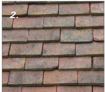
2. The most common roofing material is the red-brown clay tiles made from local Keuper Marl Clay. The clay tiles - called plain tiles - are of small scale, typically 265mm x 165mm, with a fine sand texture.
